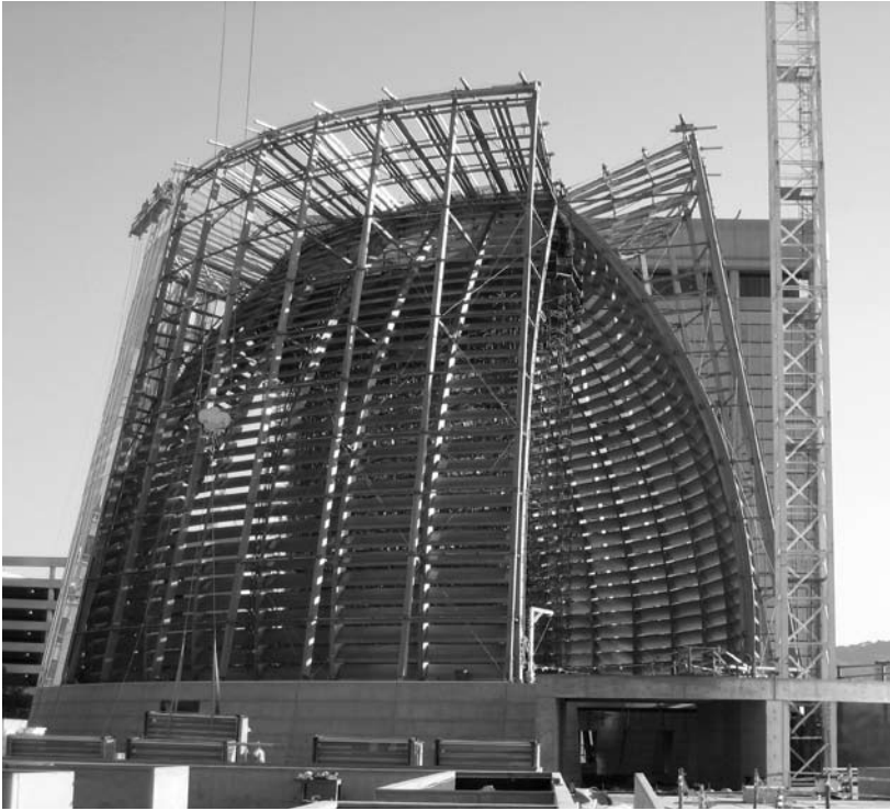
Cathedral of Christ the Light in Oakland, CA is unlike any structure in the world. The inner chords are made with (26) 10 3/4" curved glulam ribs, roughly 100' in length and varying in depth from 30" at the base to 19 1/2" at the top.
